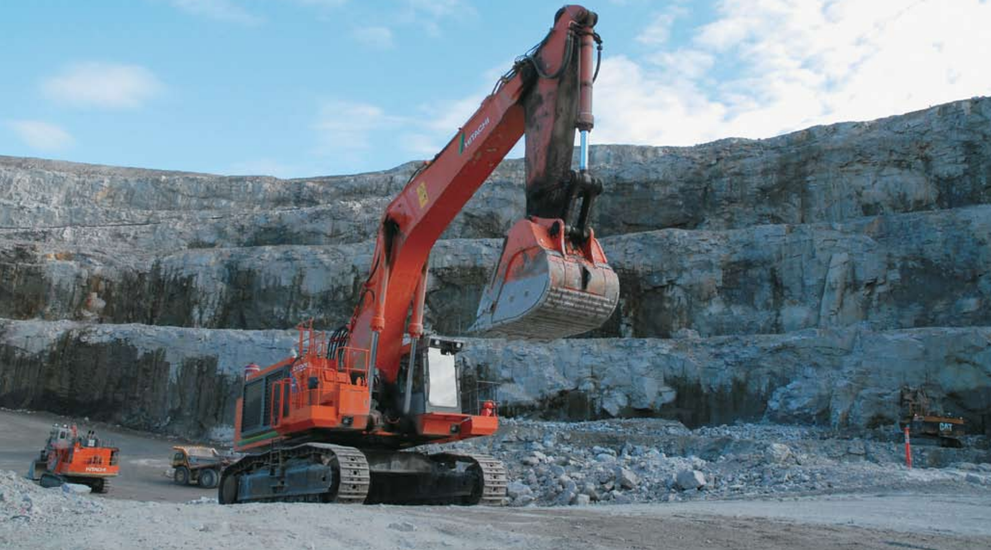
DOWN IN THE HOLE: The A154 pit has been the backbone of the Diavik operation from the start. Here, the Hitachi EX 1900 excavator, with a 22-tonne payload, repositions in the pit.
